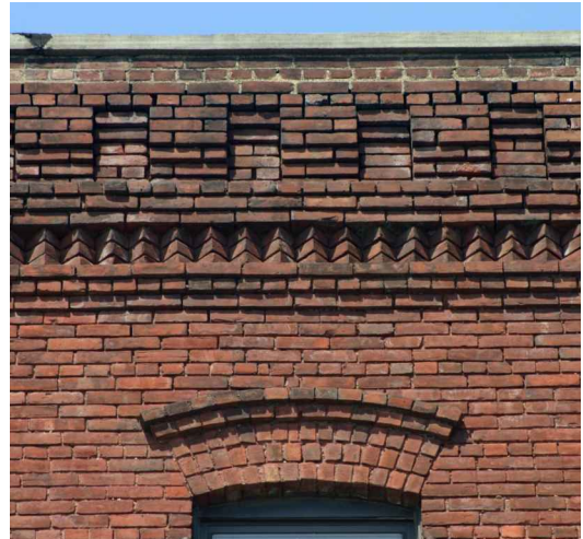
Visible open mortar joints in a corbeled brick cornice need to be repointed.
