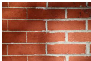
The left side of this photograph demonstrates appropriate re-pointing, whereas the right side demonstrates inappropriate re-pointing.
